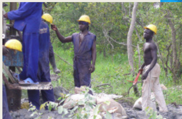
Building a new well at the site of the new Diocesan Center.
